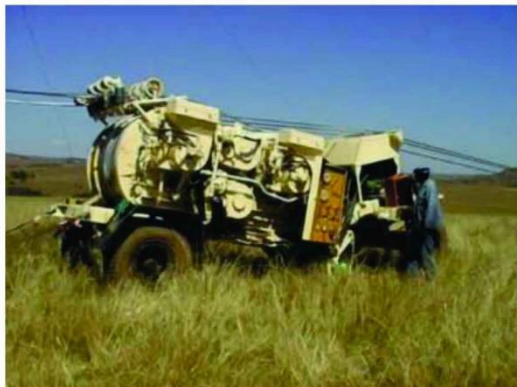
Typical example of tensioner station
